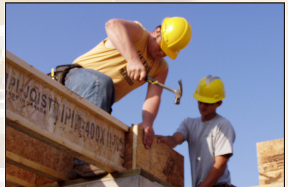
Hands-on learning experience makes a difference to employers seeking to employ framers and other construction workers.
